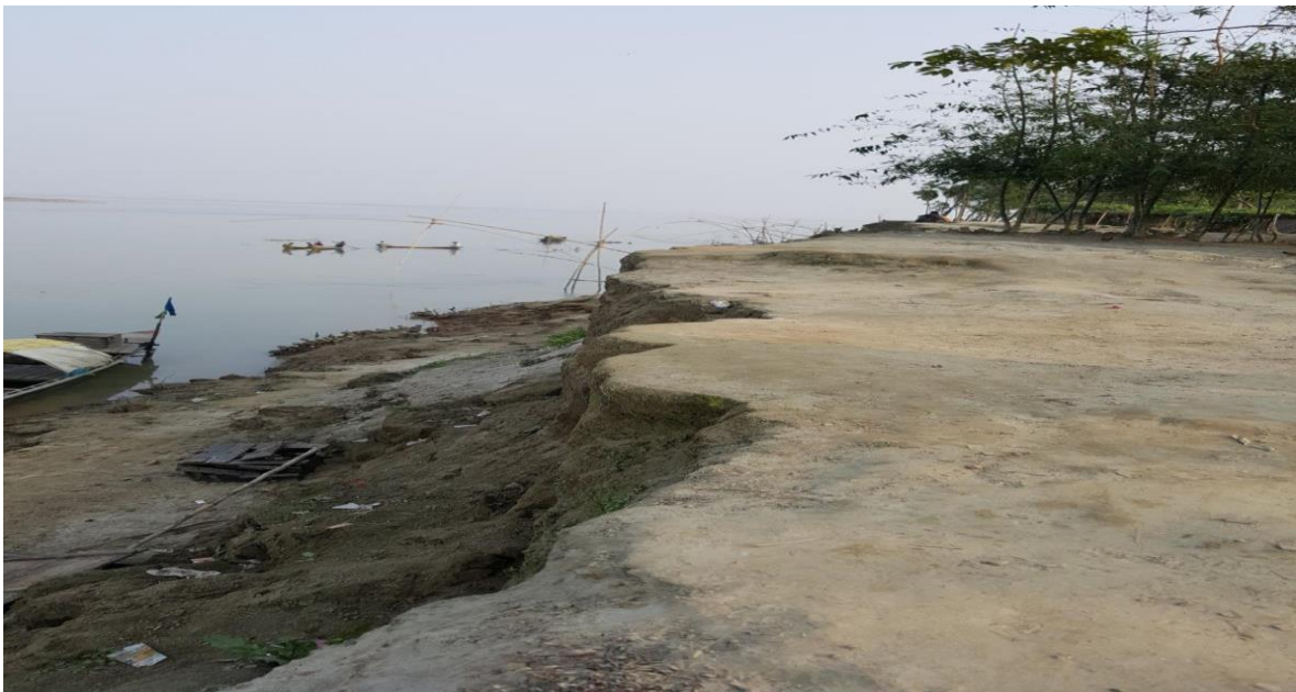
Picture: Unsafe riverbank
